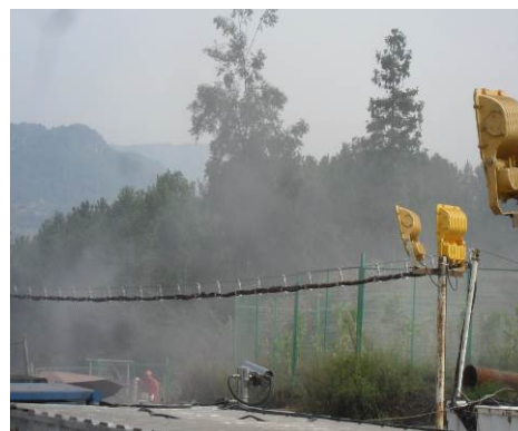
Fig.1 Separate sands by foundation trench (left), and the pollution (right).
