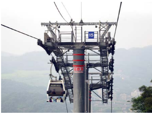
Fig. 7 An example of the damping rings (the red rings near the top of the tower) applied to the Maokong Gondola towers in Taiwan.
